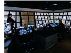
Central control room.
