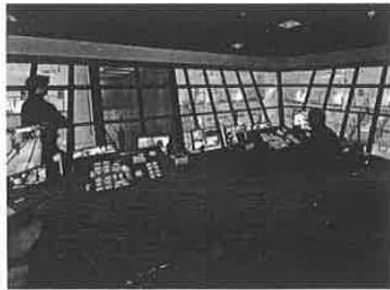
Central control room.
