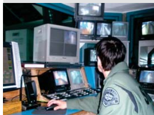
Existing central control room.
