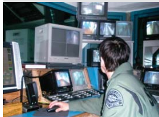
Existing central control room.
