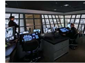
Central control room.
